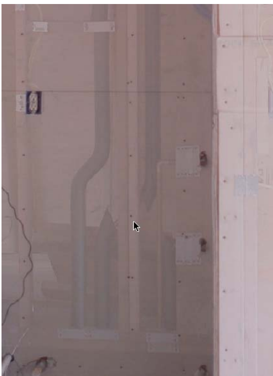
Figure 9 – “X-Ray” view of nail (at arrow) near insulated copper water pipe passing through double stud.
